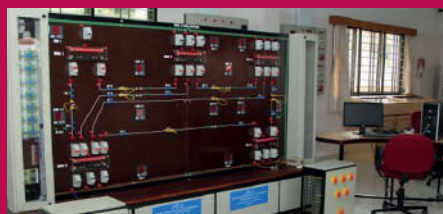
POWER SYSTEMS LAB
