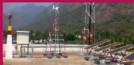
ROOFTOP RE LAB
